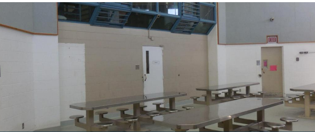
A guard booth overlooks the dining area at the N.A. Chaderjian Youth Correctional Facility
